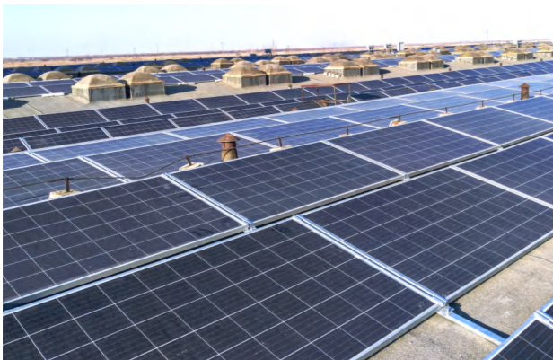
Capacity: 3MWp Location: Hebei, China Application: V-Top Rooftop
