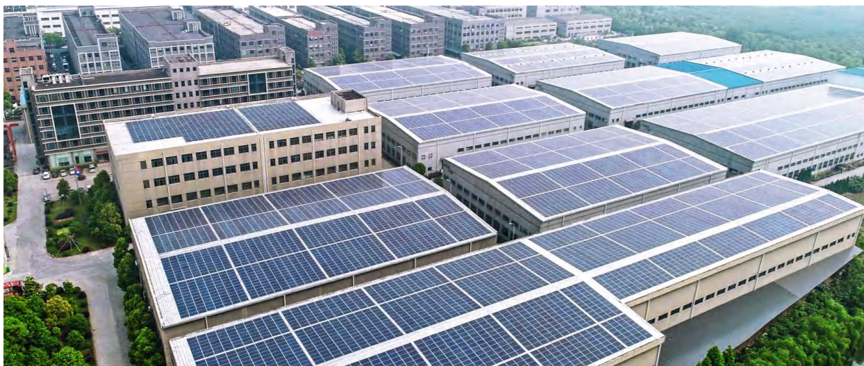
Capacity: 6MWp Location: Hangzhou,China
