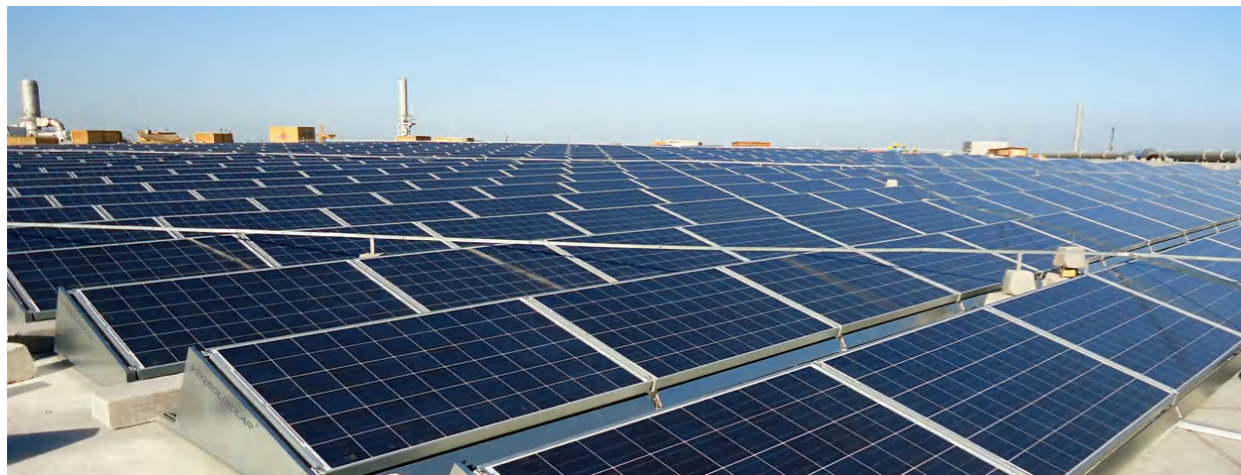
Capacity: 2MWp Location: BeiJing
