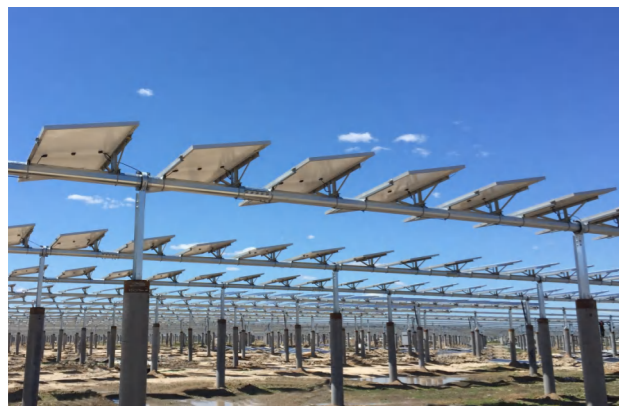
Capacity: 100MWp Location: Jilin, China Application: V-Link Tracker
