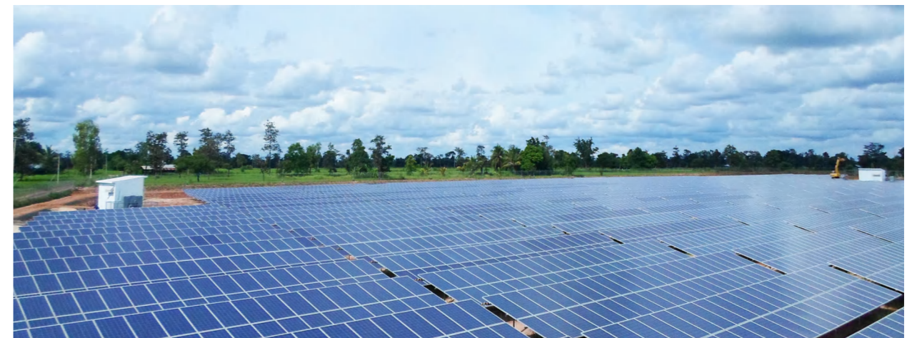
Capacity: 70MWp Location: Thailand
