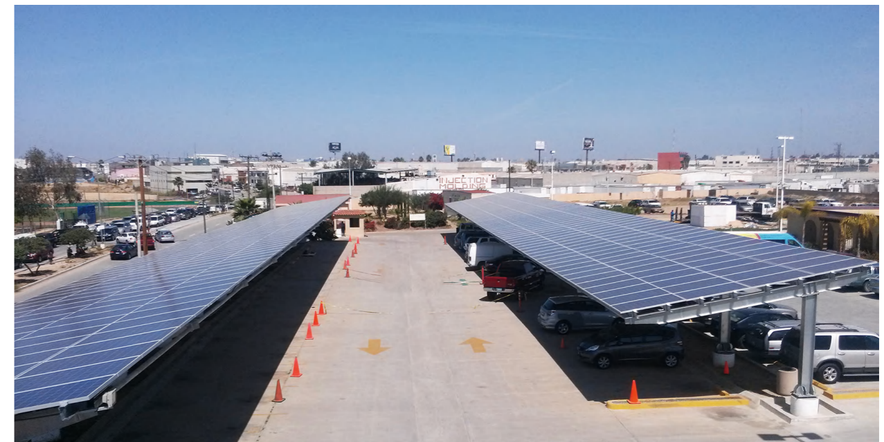
Capacity: 1MWp Location: Mexico
