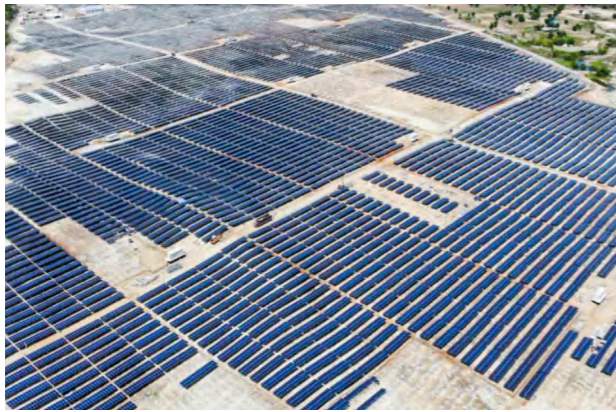
Capacity: 50MWp Location: Vietnam Application: Fixed ground photovoltaic mounting structure
